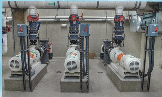
▲ The three main pumps push the water at a rate of approximately 2,640 gallons a minute.
